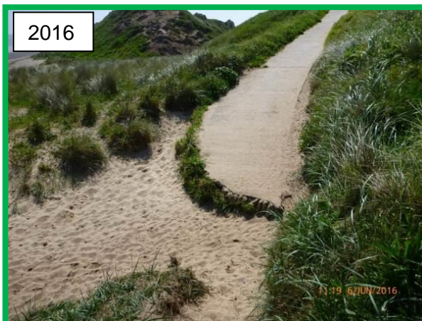
Exposure of timber piles at foot of concrete footpath (CBU E52/6)
