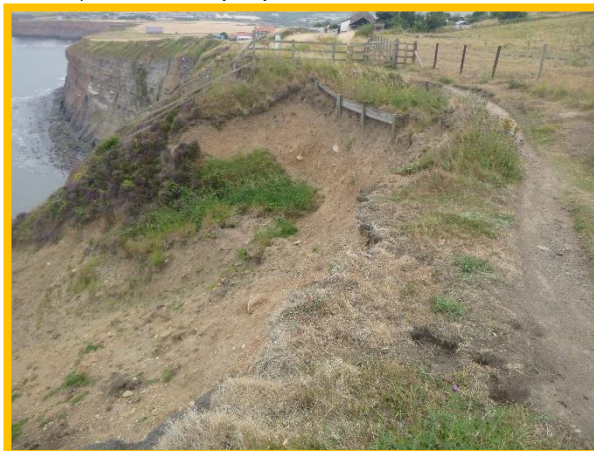
E58/1a headscarp recession encroaching on footpath.
