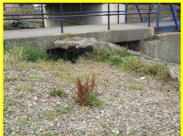
Undercutting of rock revetment apron (/C0704C06)
