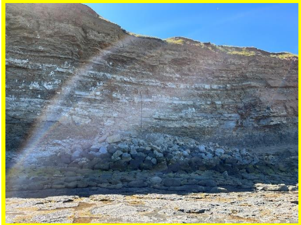
E60/1b Rock armour located at toe of cliff to the north of Cowbar Cottages
