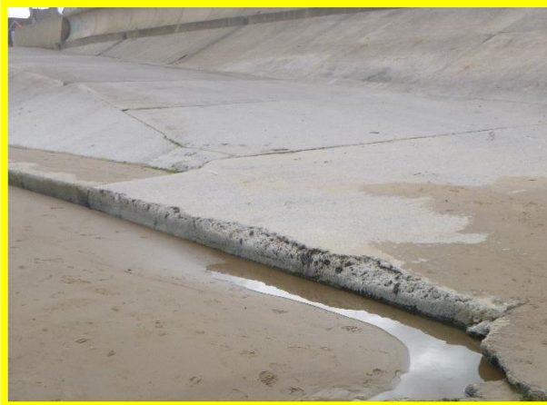
South eastern access ramp. Loss of concrete render exposing gouted stone fill beneath concrete deck slab (/C0602C01).
