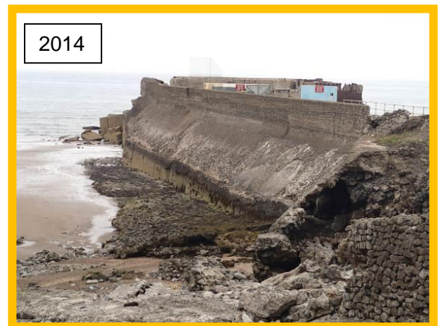
Voiding and collapse of west side of jetty structure in 2014 (Asset Ref No. 1221D901D0201C02)
