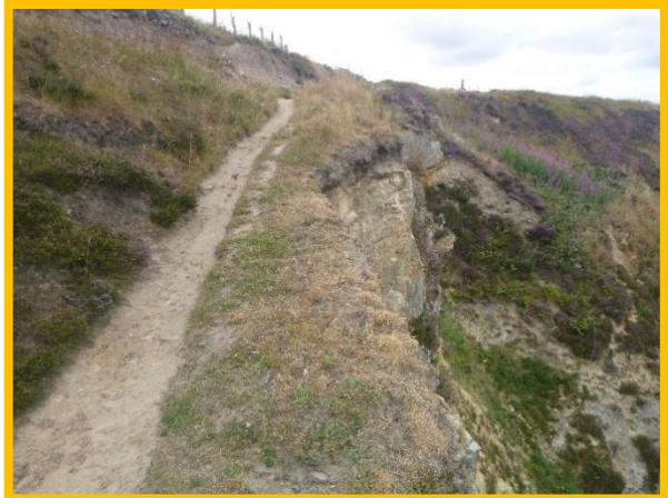
E58/5 Upper further signs of headscarp recession presenting an imminent risk to footpath stability.
