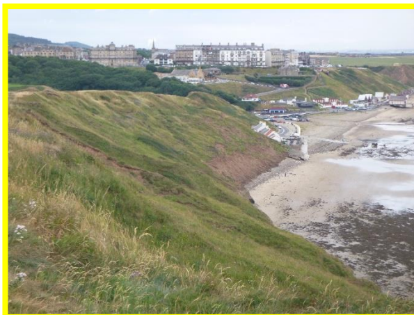
E53/3 to E53/5 Generally small-scale slumping in the till layer of the cliff northeast of Saltburn (Locally Active in August 2022).
