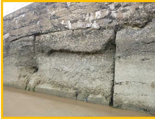
Large void visible halfway along inner face of breakwater. (Asset Ref No. 1221D901D0201C02)
