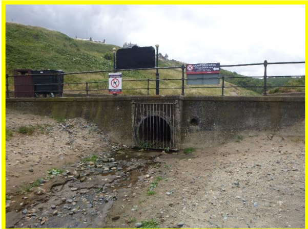
Security grille damaged (/C0703C02). Note accumulation of beach sediment around base of outfall.
