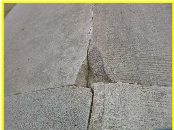
Cracking and damage to corner of slab on slipway (/C0602C01).
