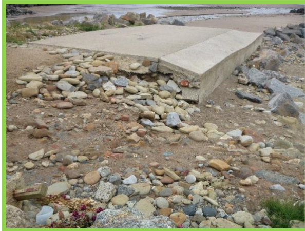
Outflanking of concrete slipway (Asset Ref No. 1221D901D0202C05)
