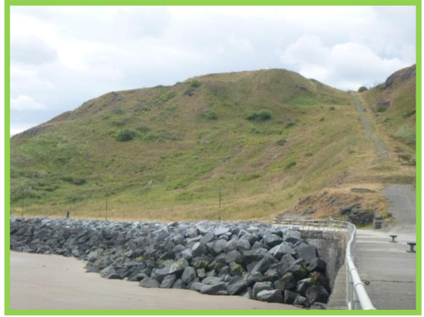
Modified rock revetment protecting inner face of jetty (Asset Ref No. 1221D901D0202C01)
