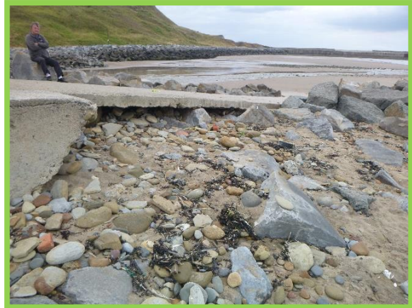
Undercutting of concrete slipway (Asset Ref No. 1221D901D0202C05)
