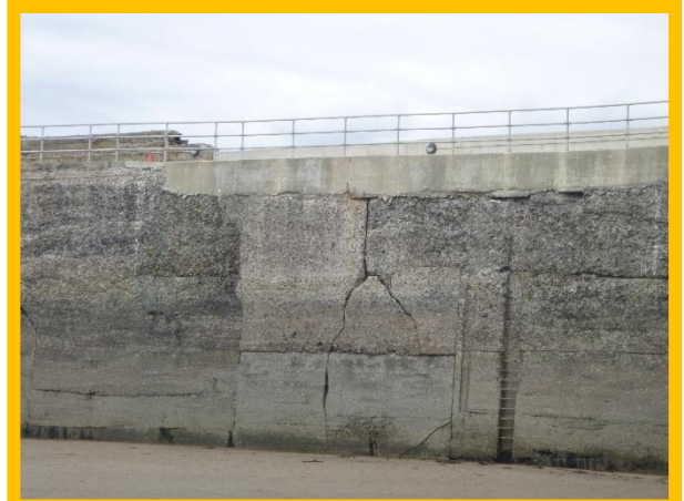
Large wishbone shaped crack on inner face of breakwater (Asset Ref No. 1221D901D0201C02)
