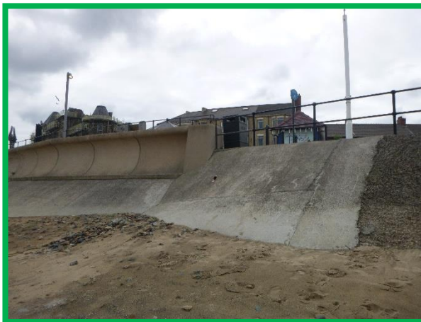
Mass concrete transition in fair condition. Note; horizontal and vertical cracks and damaged drain outfall (/C0602C06)
