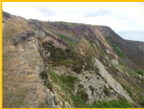
E58/2 Upper showing signs of ongoing headscarp recession. Coast Protection Asset Condition Assessment
