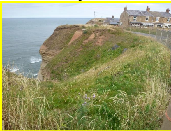
E60/1 netting has been placed on the upper till slope adjacent Cowbar Cottages to locally decrease the rate of erosion.
