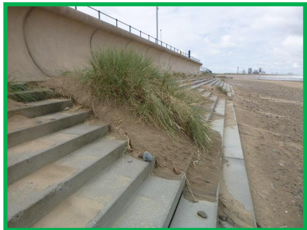
Vegetation growth on stepped revetment. (/C0602C06)
