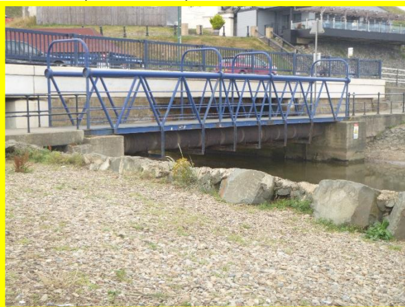
Exposed crest of grouted rock revetment to south of rock revetment (/C0704C06)
