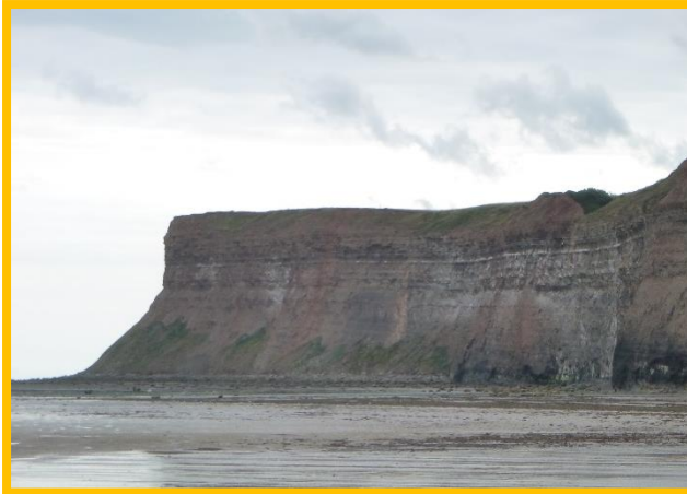
E53/1 (left) Locally Active in 2020 due to a more stable headscarp and upper slope.
