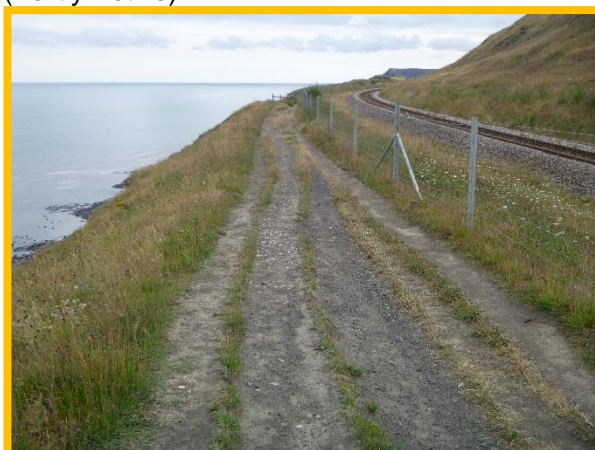
E54/3b unguarded section of footpath Hunt Cliff showing active cliff face and debris apron (Partly Active)
