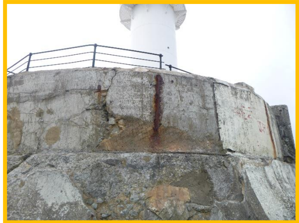
Northern extent of upper structure in poor condition (/C0506C01)
