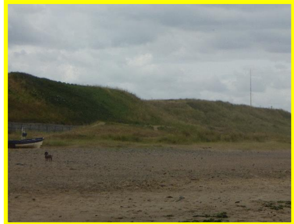
Evidence of recent shallow seated slips CBU E52/8
