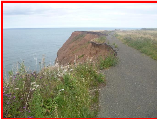
E59/4 Ongoing erosion of soft till layer leading to collapse of road (Totally Active).
