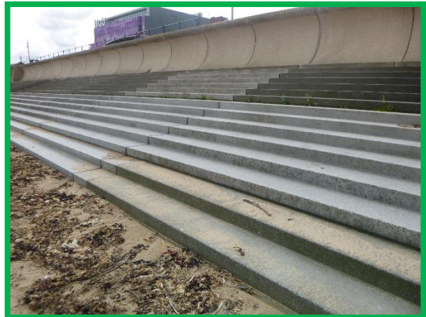
Evidence of repaired sections of the stepped concrete revetment in good condition (/C0602C02)
