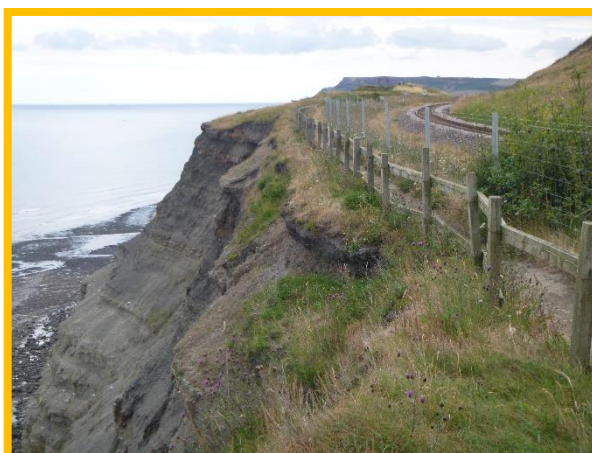
E54/3a proximity of footpath and railway line to actively eroding cliff top (Partly Active)
