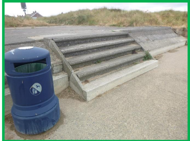
Recently repaired step at The Stray (/C0603C01)
