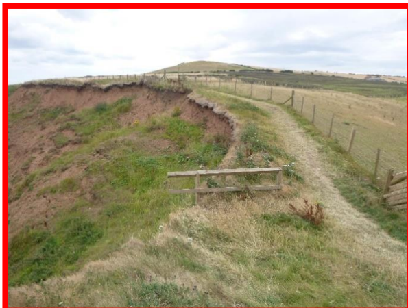
E57/7 Slumping and recession along headscarp (Totally Active)
