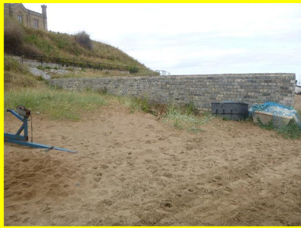
High beach levels obscure masonry wave wall and north west of beach entrance (/C0702C02)
