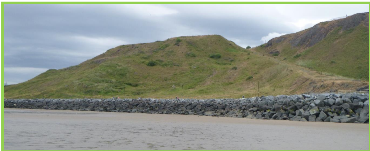
General view of rock armour revetment in 2022. Good profile and interlock. (Asset Ref No. 1221D901D0202C01)
