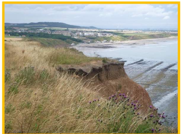
E53/2 Ongoing headscarf recession with some slumping of the till layer of the cliff northeast of Saltburn (Partly Active)
