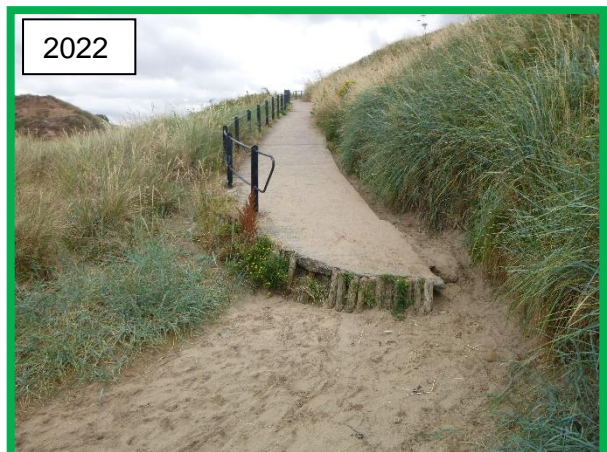
Further exposure of timber piles at foot of concrete footpath (CBU E52/6)
