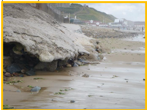
Undercutting and voiding in mass concrete apron (/C0704C05)
