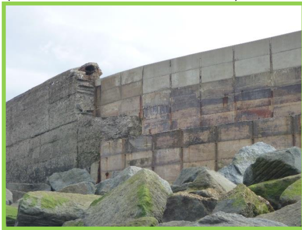
Seaward face of repair. Exposed re-bar and corrosion staining (Asset Ref No. 1221D901D0201C02)
