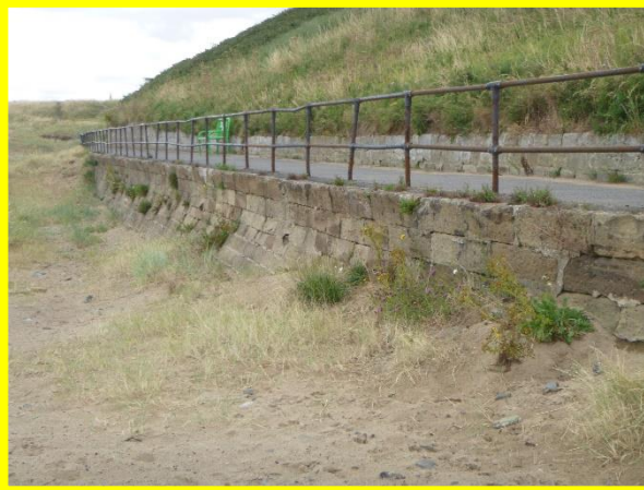
Wall in fair condition some missing mortar and open joints (/C0702C03)
