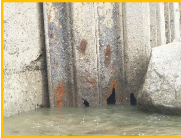
Void visible In base of sheet pile at seaward end of structure (Asset Ref No. 1221D901D0201C02)
