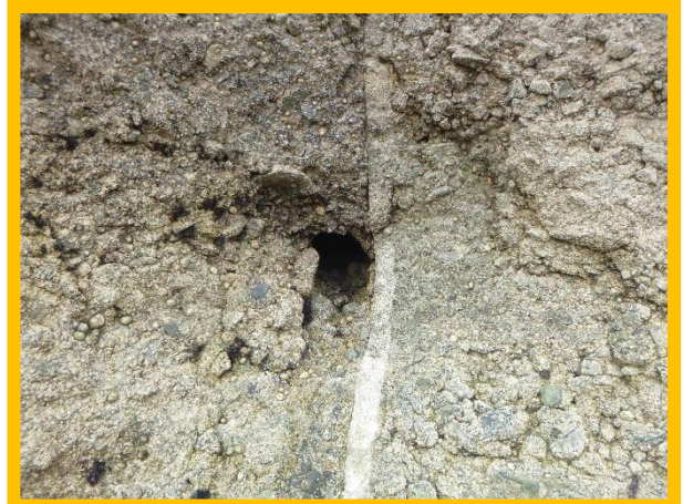
Close up of hole in void (Asset Ref No. 1221D901D0201C02)
