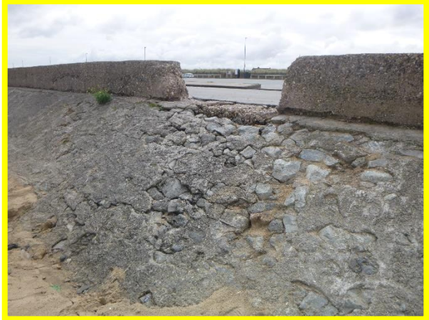
Gap in concrete visible (/C0601C01)
