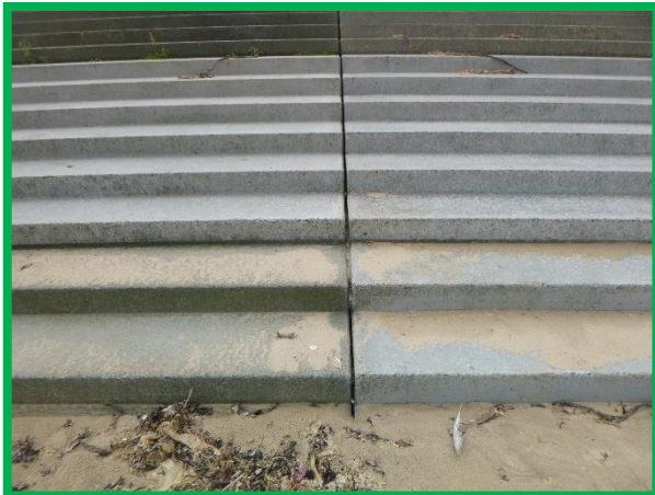
Open joints in stepped concrete revetment. Overall condition remains as very good (/C0602C02)
