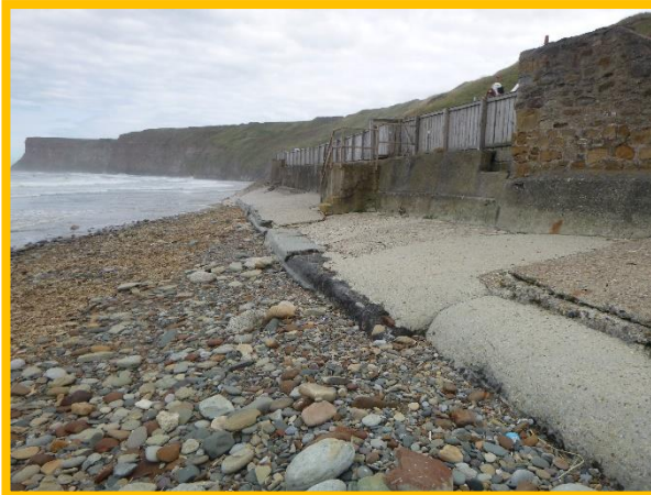
Undercutting of concrete apron (/C0704C05)
