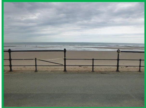
Damage to handrailing along promenade (/C0702C04)
