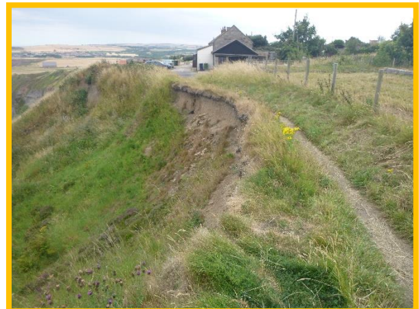
E58/1a headscarp recession encroaching on footpath.
