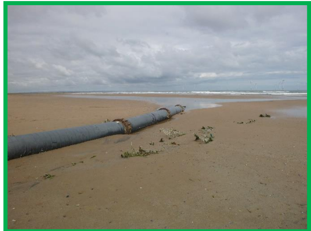
Outfall on Coatham Sands in poor condition, beach levels higher than 2020 (/C0507C01)
