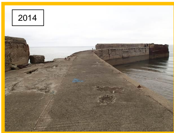
View of crest from access gate showing missing section of crest wall and damaged deck in 2014 (Asset Ref No. 1221D901D0201C02)
