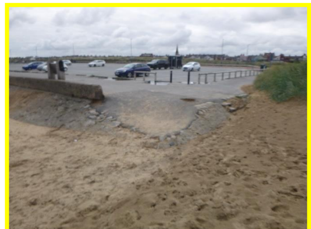
High beach levels have covered previously recorded undercutting of western corner of the asset (/C0601C01)
