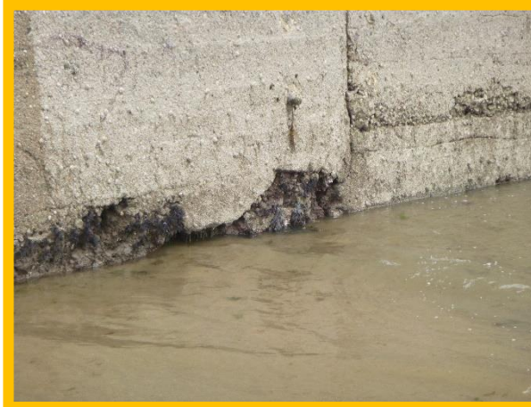
Scour visible at base of breakwater (Asset Ref No. 1221D901D0201C02)
