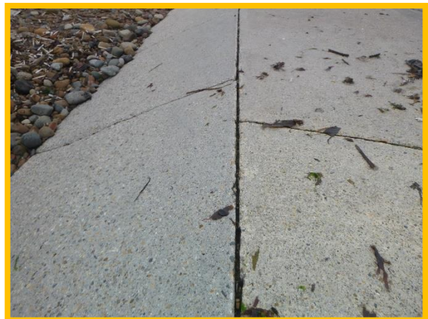
Open joints missing sealant (/C0704C05)
