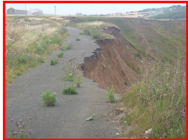
E59/3 Ongoing erosion of soft till layer leading to collapse of road (Totally Active).
