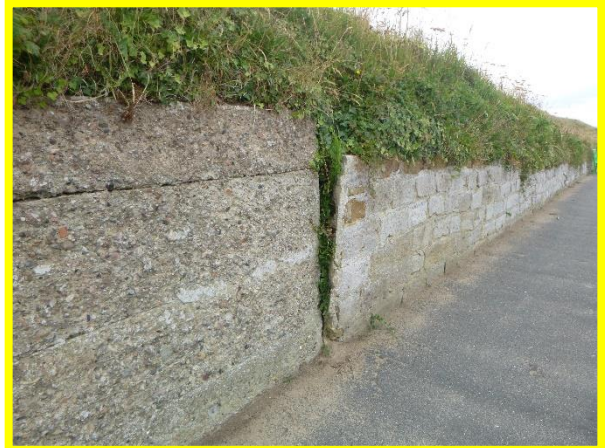
Masonry wall showing signs of lateral movement (/C0702C03)
