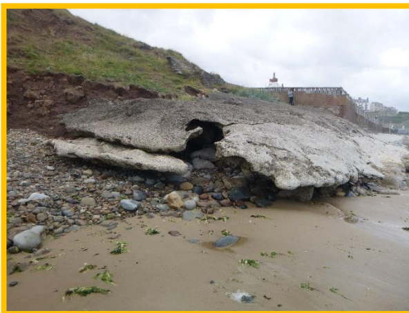
Undercutting of mass concrete apron (/C0704C05)
