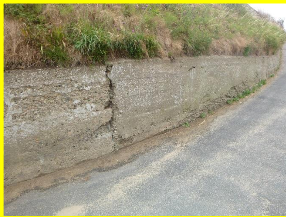
Crack in wall – no apparent change (/C0702C03)
