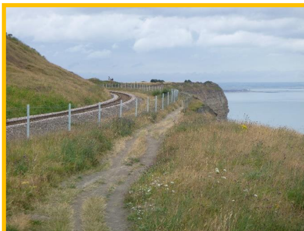
E54/2a proximity of footpath and railway line to actively eroding cliff top (Partly Active)
