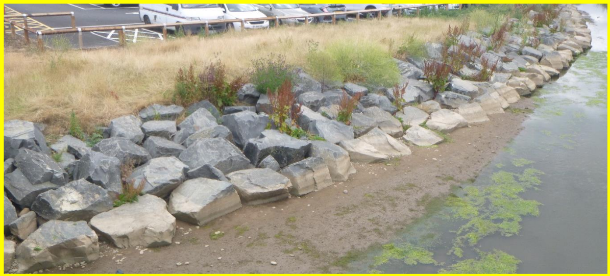
New rock armour revetment at Skelton Beck, looking upstream from the Saltburn Road bridge.
