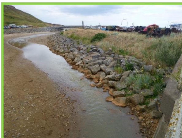
Rock armour protection along eastern edge of Kilton Beck. (Asset Ref No. 1221D901D0202C05)
