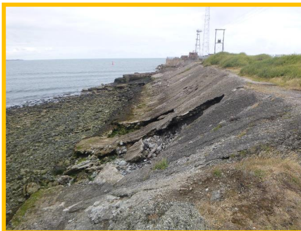
Large void in western face has worsened in 2022 (/C0506C01)
