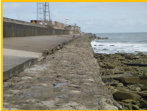
Failed coping slab along eastern face (/C0506C01)
