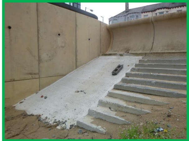
In-situ cast transition unit between stepped revetment and new cinema wall (/C0602C06) & (/C0602C05)
