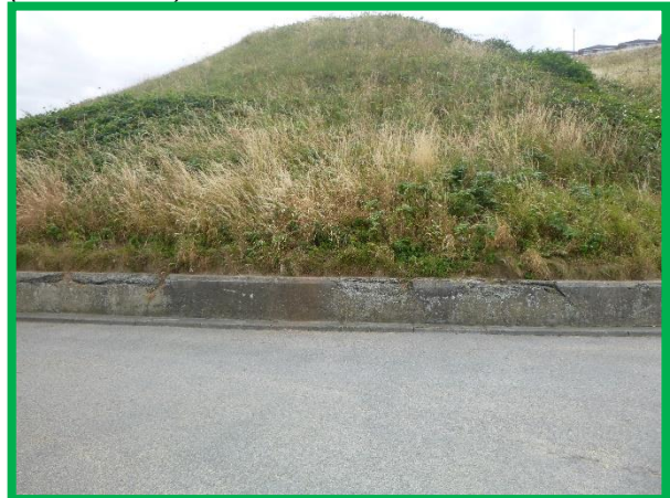
Further damage to shallow retaining wall (/C0702C04)
