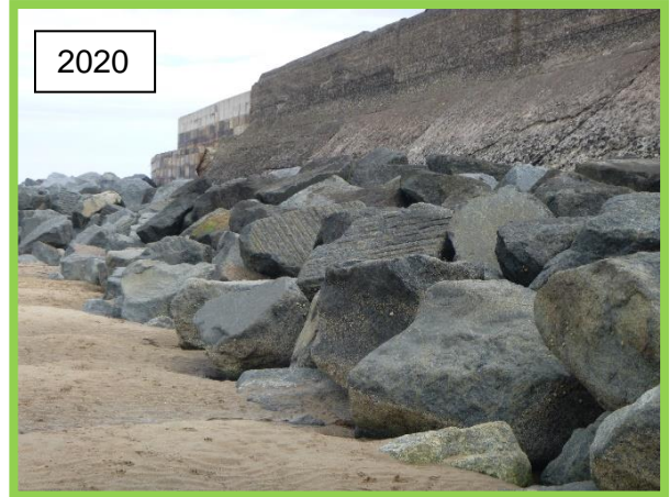
Seaward face of wall. Rock armour profile poor in places (Asset Ref No. 1221D901D0201C02)
